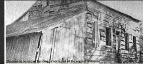
The join-to-go end of building is not a part of the original residence Lyman Wight home In Adam-ondi-Ahman
